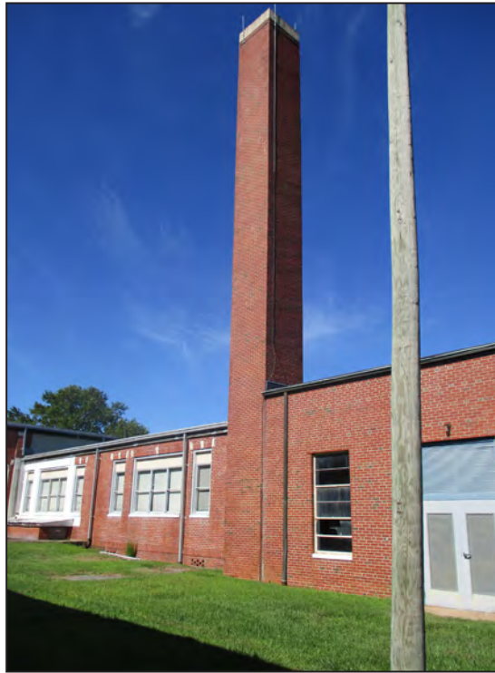
Photograph 7: View of east elevation of Front Hall and boiler room; looking southwest. (2018)
